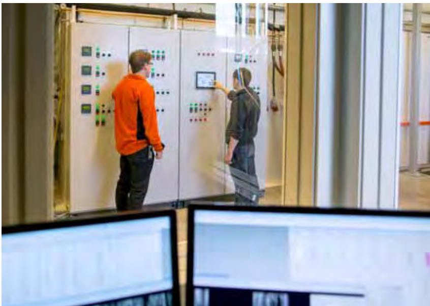
Since December 2012 a highly advanced test facility for air/water heat pumps enables the simulation of all types of climate situations when conducting function tests.
