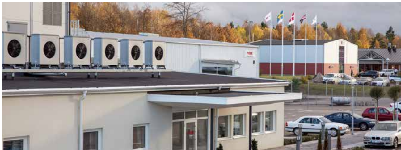
In 2012 a brand new heat-pump array was installed at the Heat-pump Plant in Markaryd. The array produces 180 kW of heat from energy taken partly from five 160-metre deep boreholes and partly from the outside air with the aid of six NIBE AMB air collectors of around 20 kW each. Energy is also recovered from the air used when function-testing products as part of the manufacturing process.
